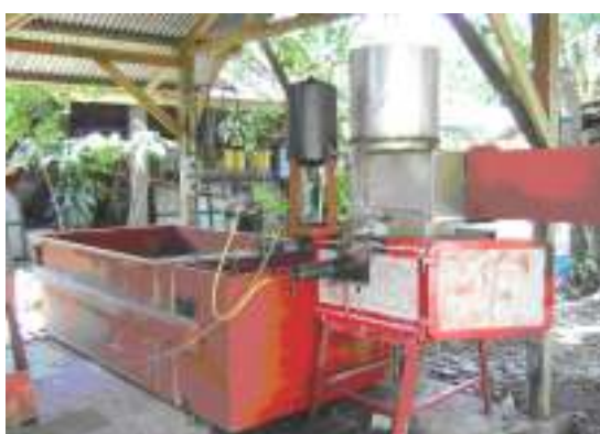
Figure 12 . Hot water tank system
