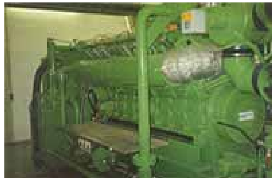
Photo 6: Co-generation unit (JMS 312)
