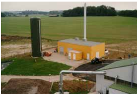
Photo 5: Bio-filter for biogas cleaning
